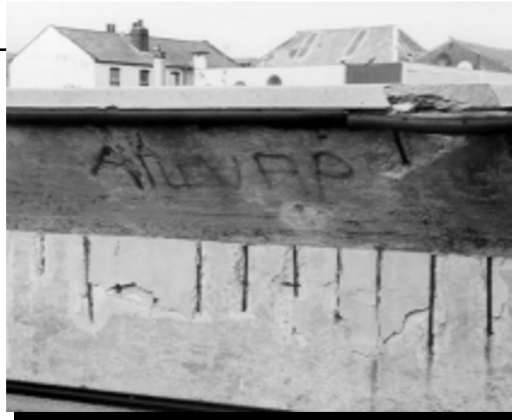
Typical low cover corrosion from carbonation
