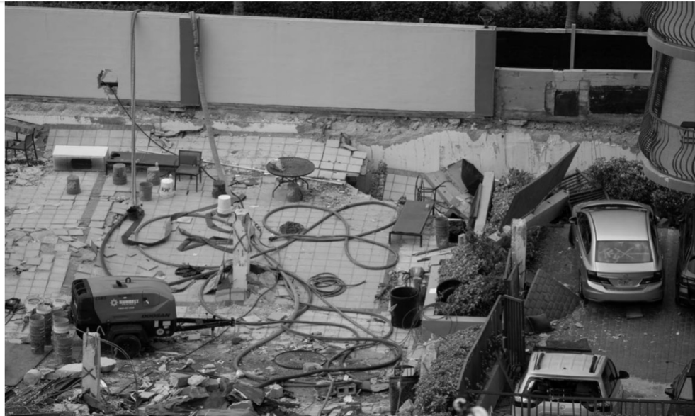
A photo of the Champlain Towers South pool deck shows the slab disconnected from the southern wall during the June 24 collapse. Damage in the failure plain is not uniform, indicating pre-existing damage to portions of the slab at the connection, according to engineer Dawn Lehman. Robert Lisman
