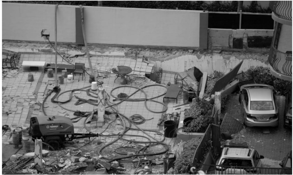
A photo of the Champlain Towers South pool deck shows the slab disconnected from the southern wall during the June 24 collapse. Damage in the failure plain is not uniform, indicating pre-existing damage to portions of the slab at the connection, according to engineer Dawn Lehman. Robert Lisman
