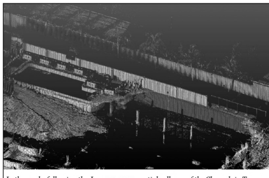
In the weeks following the June 24, 2023, partial collapse of the Champlain Towers
